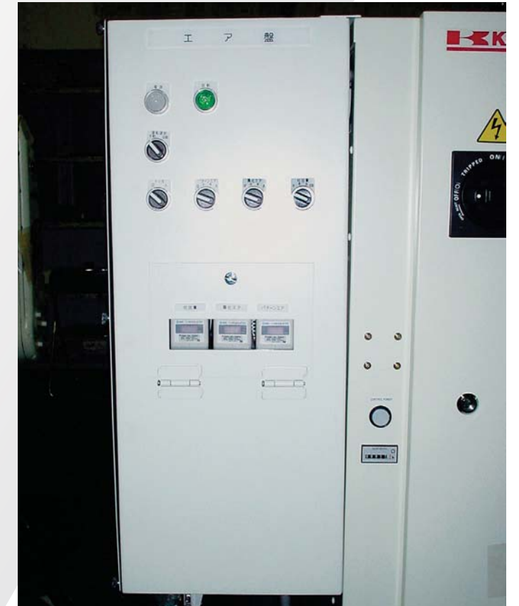
Painting unit control panel
